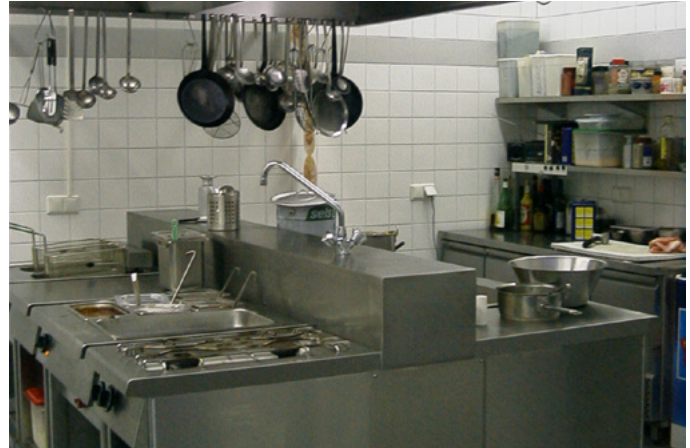
Filter monitoring in kitchens
